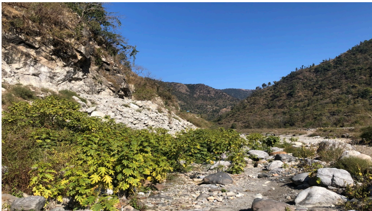
Figure C13: Study of EIA of formation cutting after one working season at a hill road in Uttarakhand
