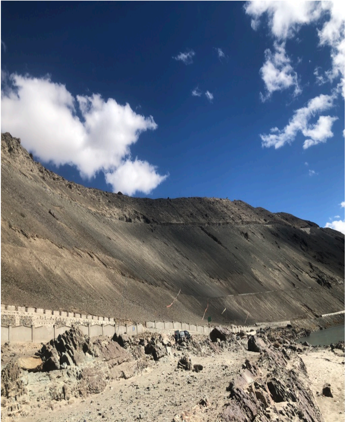
Figure 6.1 Study of retaining wall on a hill road along River Indus at Leh, Ladakh
