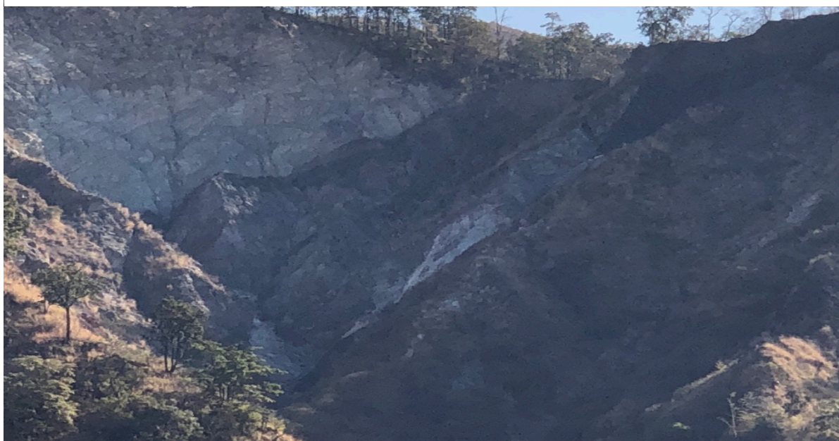
Figure C10: Studying effect of landslides on flora and fauna due to vegetation and trees getting uprooted on rural hill roads in Uttarakhand
