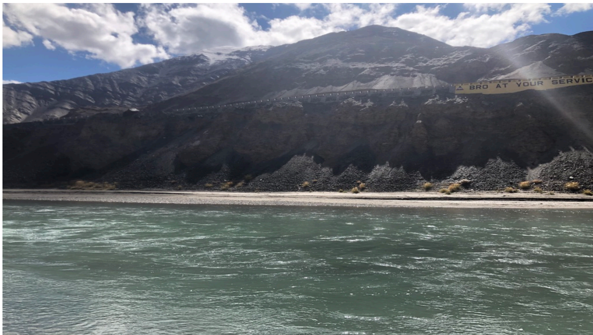
Figure C20: Scouring of hill road along River Indus at Leh, Ladakh.
