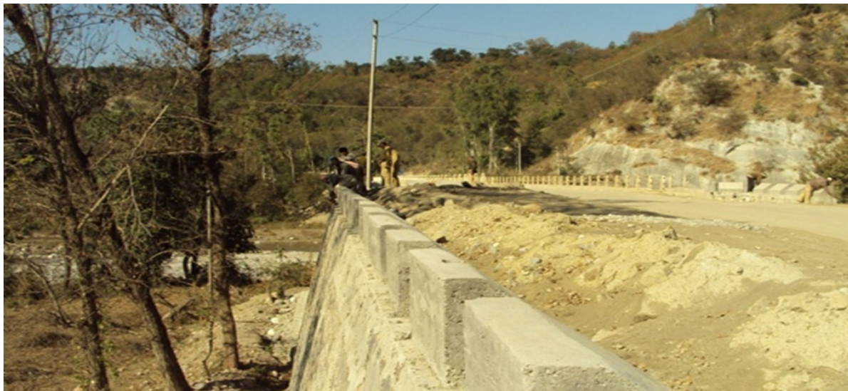
Figure 3.4 A Retaining Wall Being Constructed to Avoid Cut Section (Source: Author's Field Survey)
