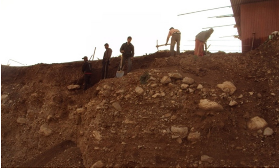
Figure 3.12 A Fresh Cut Slope Caved in due to Rains (Source: Author's Field Survey)
