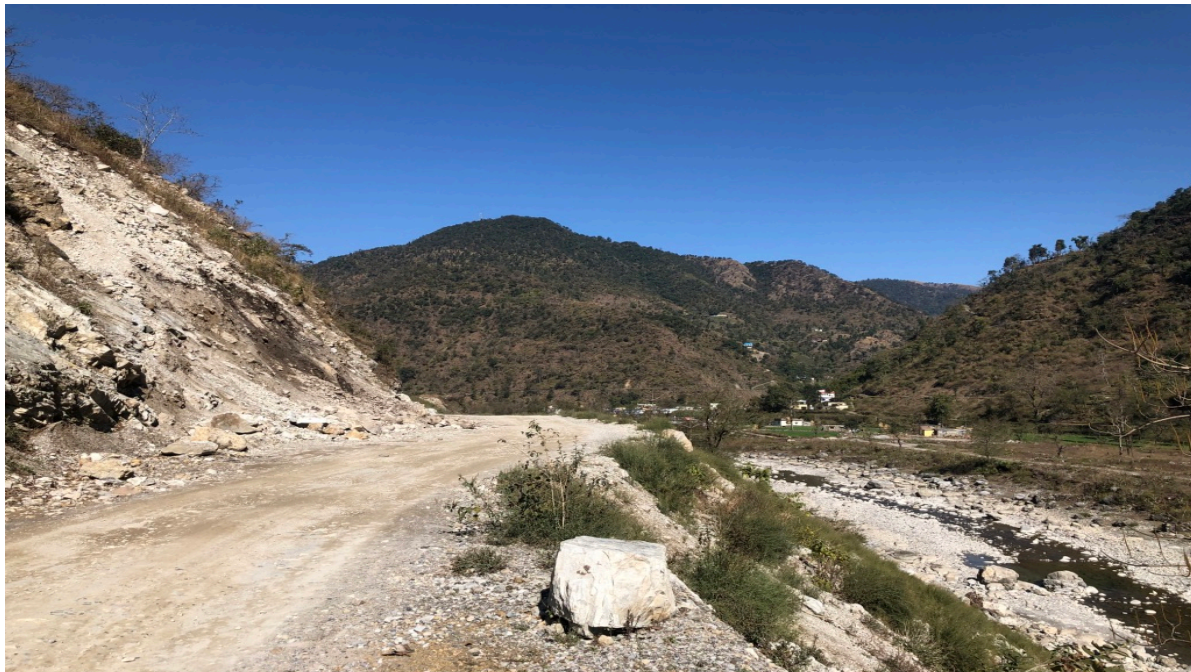
Figure C15: Study of landslides induced by unstable strata on slopes of hill road in Uttarakhand
