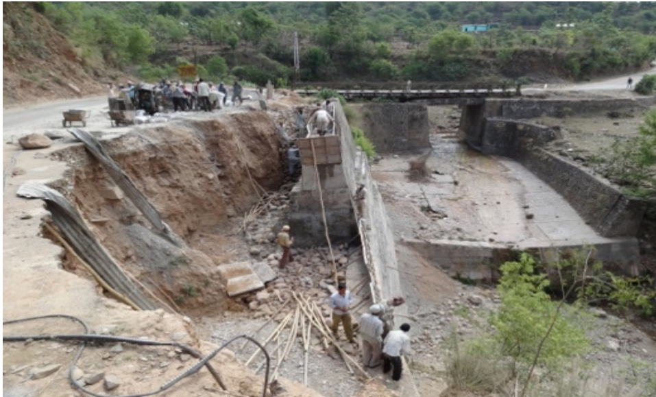
Figure 3.15 Landslide at milestone km 18 During Rainy Season (Source: Author's Field Survey)
