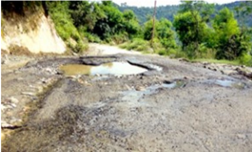
Figure 3.14 The Potholes Caused Due to Lack of Drainage (Source: Author's Field Survey)
