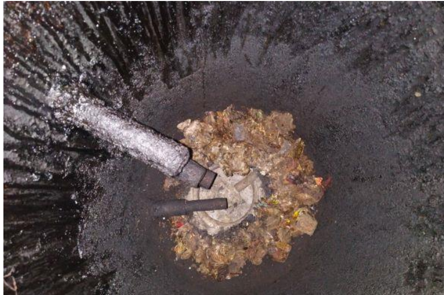
Fig. 5.25 Picture of the inside of the gasifier for the RDF pellets gasification
