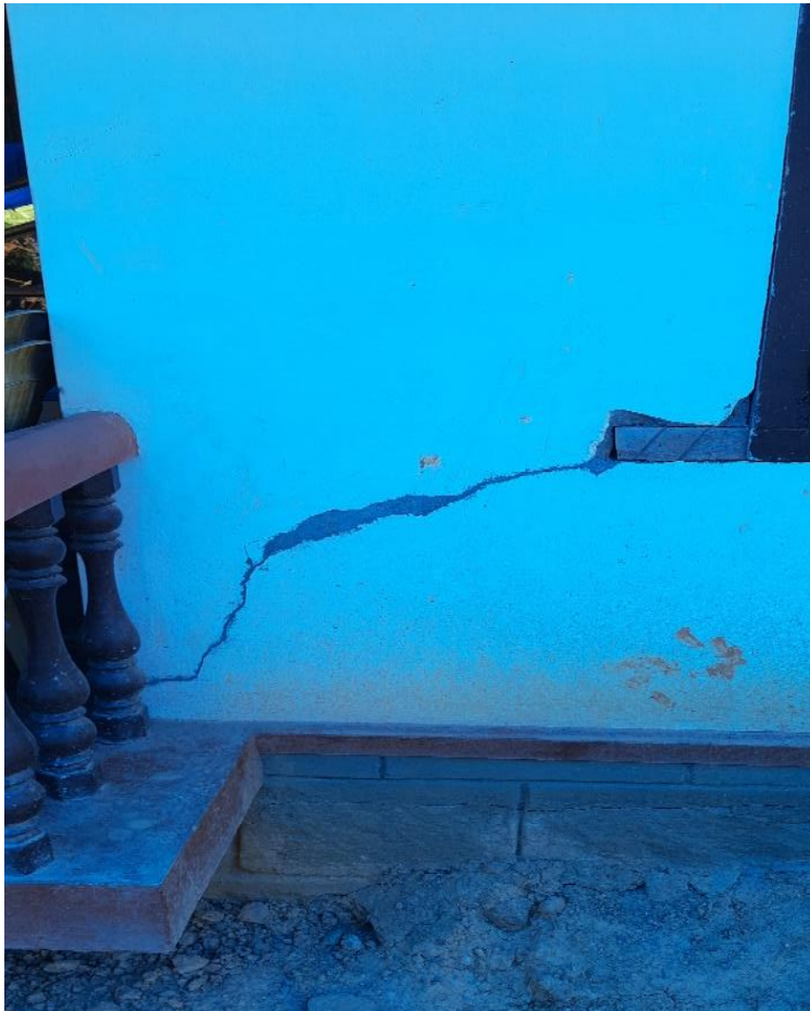
Figure 3. 5: House with cracks which is not yet rebuilt
