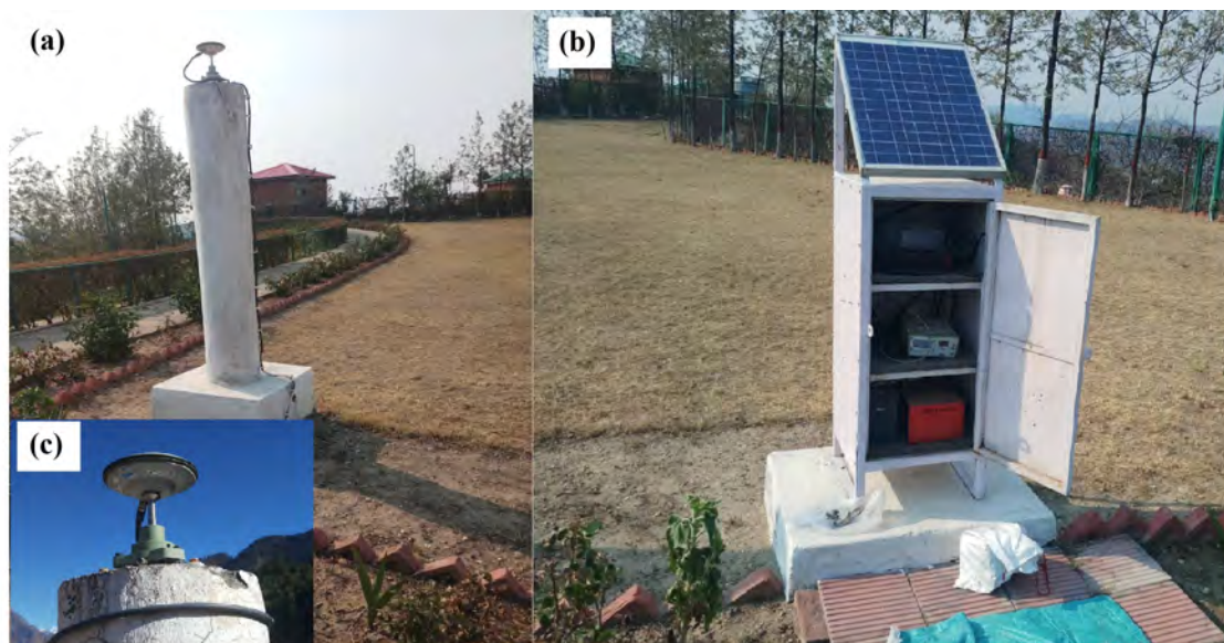
Figure 2.3: A typical setup of a continuous GPS site. (a) RCC pillar; (b) enclosure of GPS receiver, UPS power back up, internal batteries, and solar panels; and (c) GPS antenna on RCC pillar.
