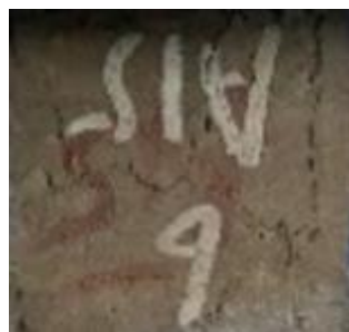
(a) Multiple cracking
