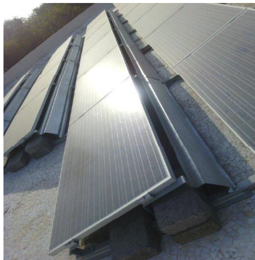
Figure 4.3 Rooftop Solar Pictures
