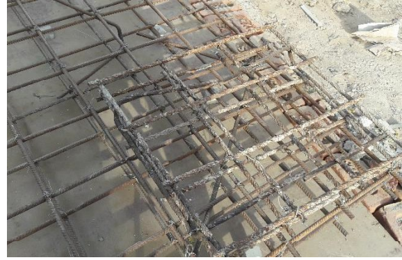
(b) Mat of corroded rebars
