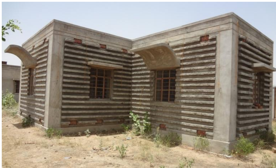
Fig. 4.14 View of room R3 (a) View of the west and south walls
