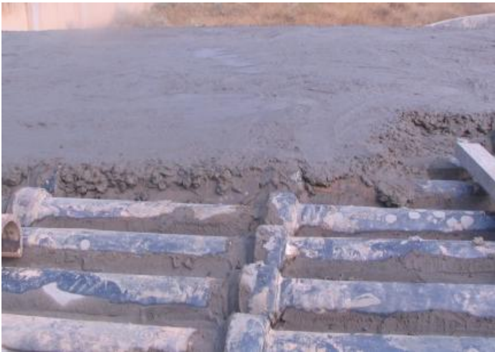
Fig. 4.17 View of hollow roof under construction (a) View of the hollow stoneware pipes (b) View of concrete layer over hollow stoneware pipes
