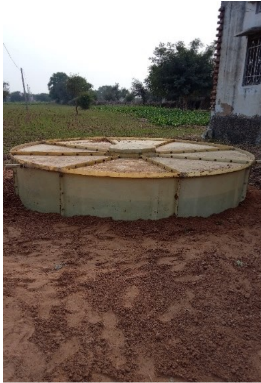
Figure 6. 8 Installed household tank
