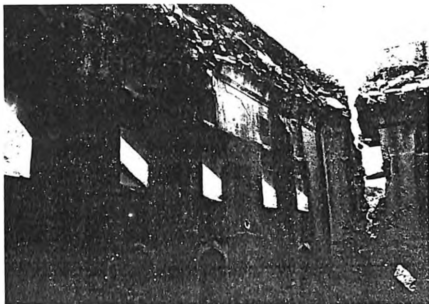
Dilapidated condition of a rear room in the 18th Century temple complex in Kanak Vrindavan valley.
