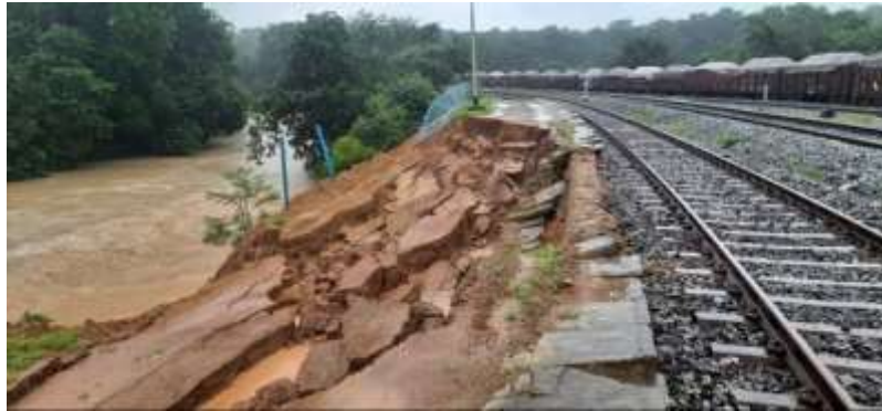
Figure 1.1 Railway embankment failure due to rainfall in Belgavi, Karnataka, India (Deccan Herald, August 17, 2020)
