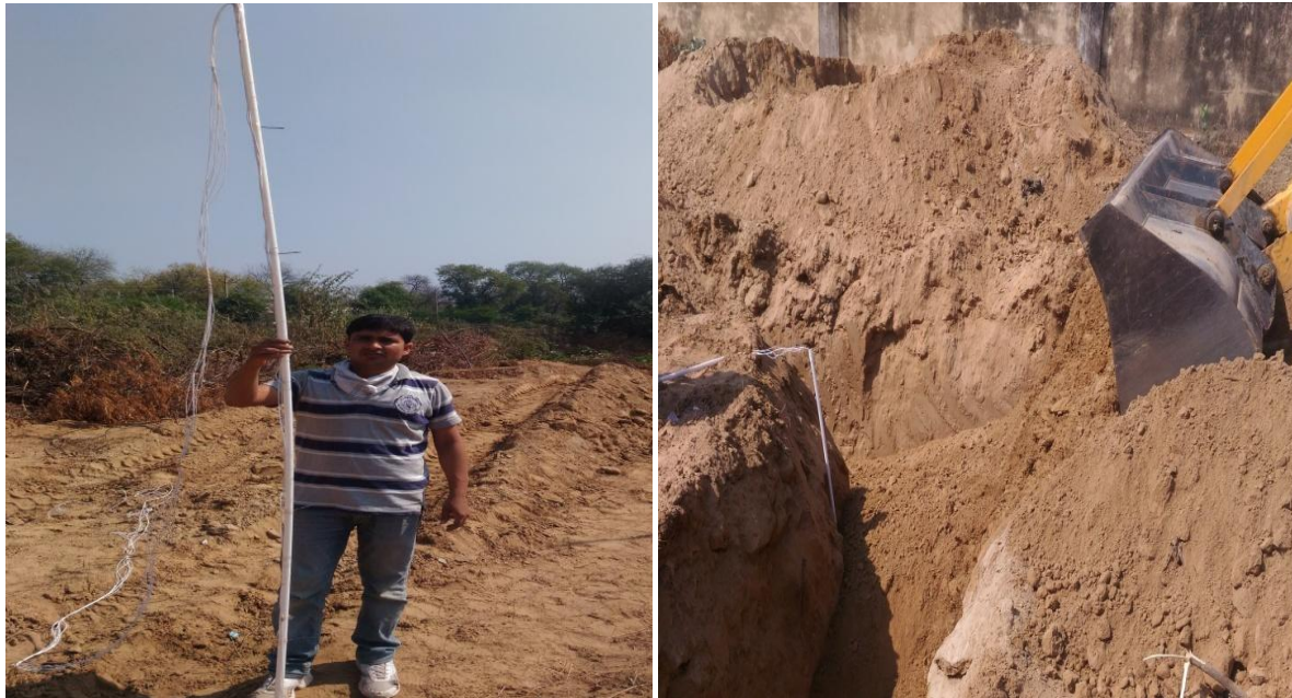
Fig. 4.10 Installation of RTDs at various depth of soil from the ground surface
