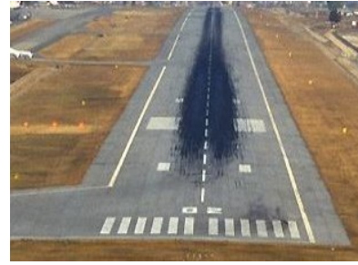
(c) Rubber deposition on runway
