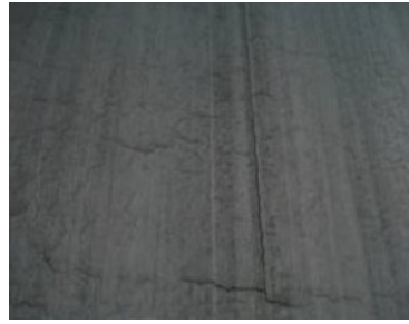
(b) Cracks on runway
