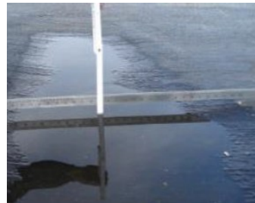
(b) Rutting on exit taxiway ET2
