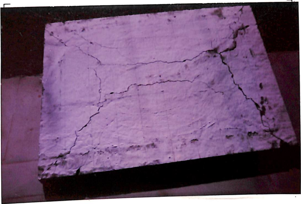
Fig.7.7 Crack pattern of Solid Slab
