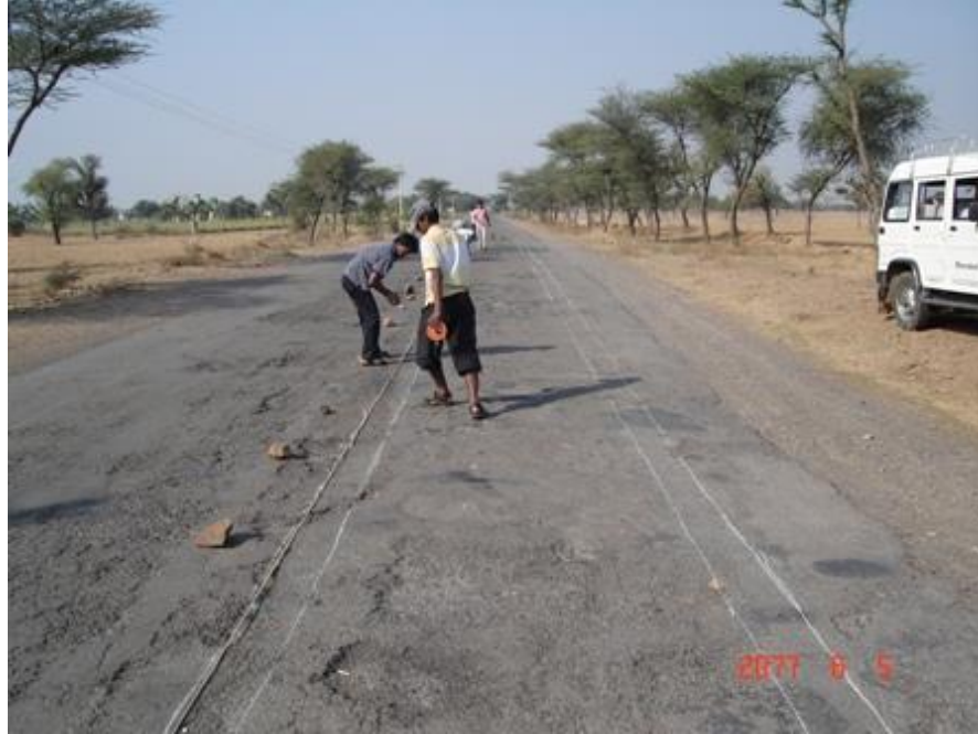
Plate 4.1: Marking along the Wheel Path
